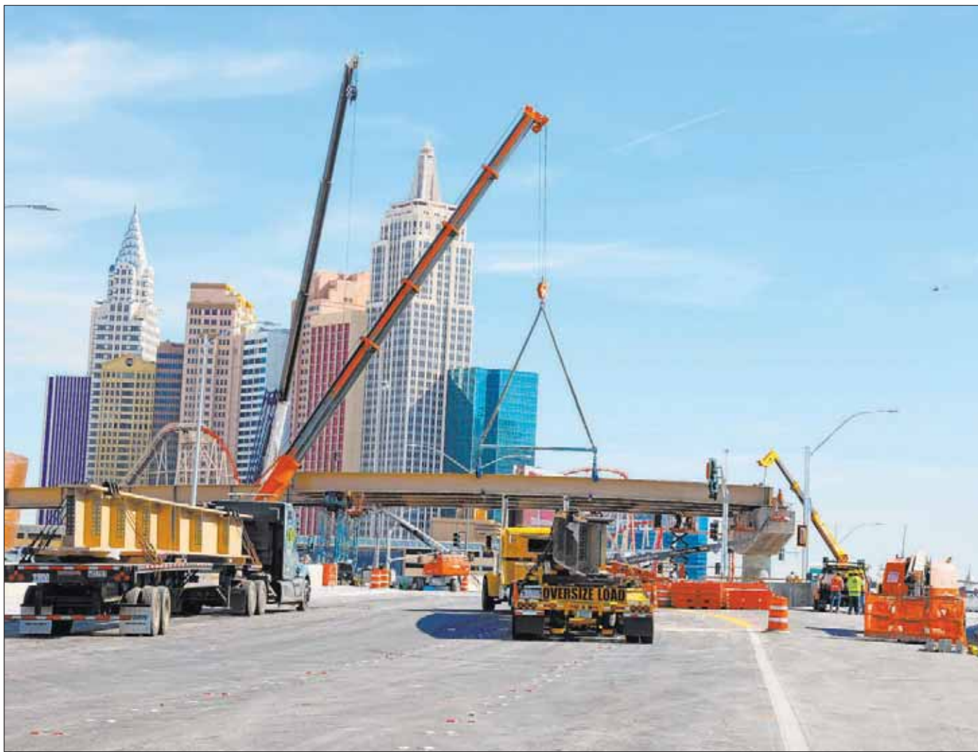
Construction continues to connect the Tropicana Avenue exit ramp on Interstate 15, as part of the Interstate 15-Tropicana interchange project. The diverging diamond interchange lane system on the Tropicana bridge will return Tuesday morning.
